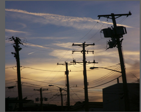
Some/ A lot of overhead wiring
